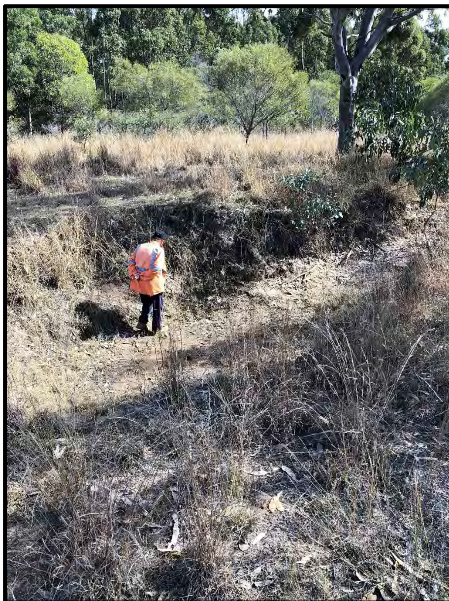
Eroded drainage channel at HVO-1199
